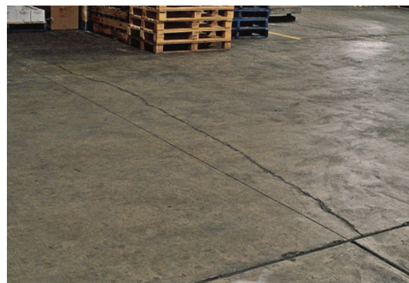
Figure 2.32 Crack adjacent to joint due to dowel 'lock-up'
