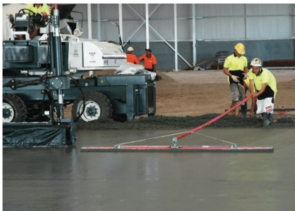
Figure 2.18 Use of wide bullfloat or 'bump cutter' in transverse direction to improve flatness of surface
