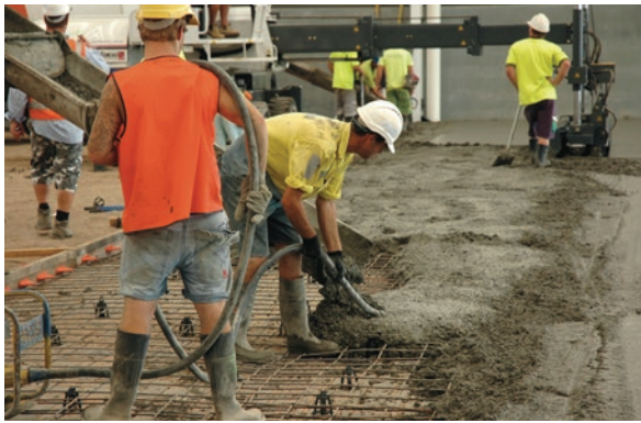
Figure 2.10 Poker vibrator used to compact concrete for thick slab prior to use of vibrating screed
