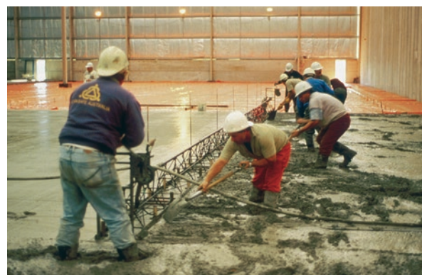
Figure 2.14 Base being compacted with a double vibrating truss beam (note the height of concrete is not more than 50-mm above finished level)
