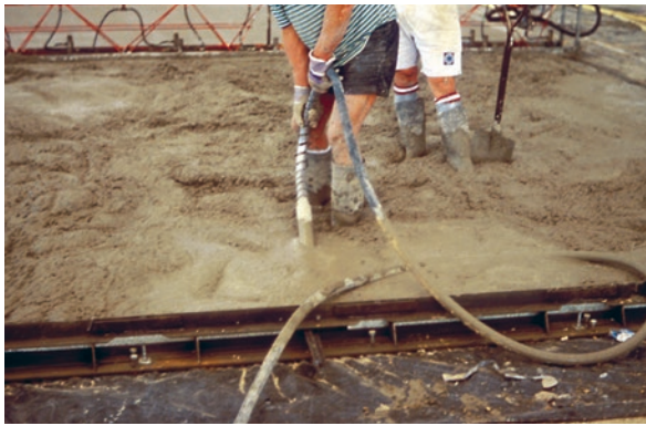
Figure 2.15 Poker vibrator being used to compact concrete near base edges, ahead of vibrating beam
