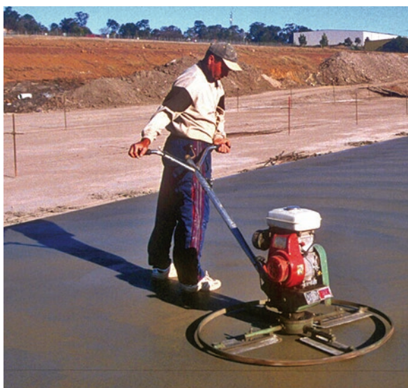
Figure 2.22 Pavements exposed to rapid drying may leave insufficient time for trowelling and work area should be reduced or number of trowels increased
