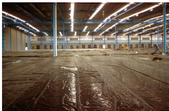
Figure 2.27 Plastic sheeting used for curing – sheets must be lapped and weighed down or secured at edges
