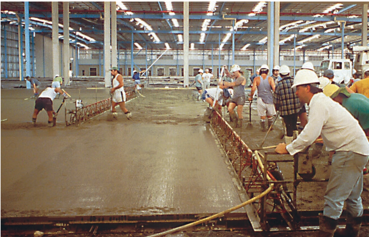
Figure 2.5 Temporary screed rails used to support vibrating truss screeds (rails are removed and void filled as work proceeds).
