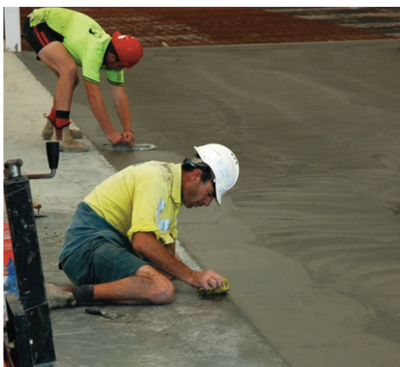
Figure 2.20 Finish near edge being improved with a steel hand trowel and cleaning of existing surface to ensure levels match
