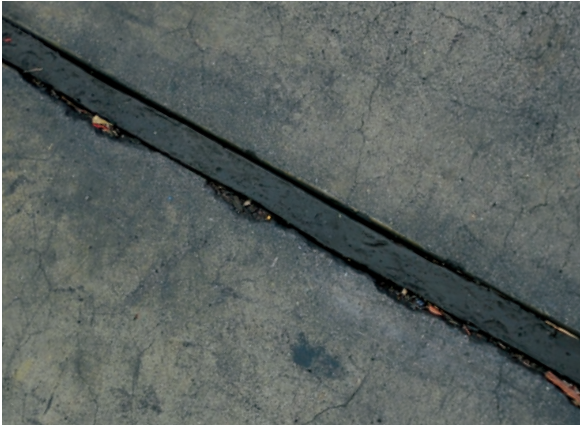
Figure 1.13 Failure of sealant at interface with the concrete
